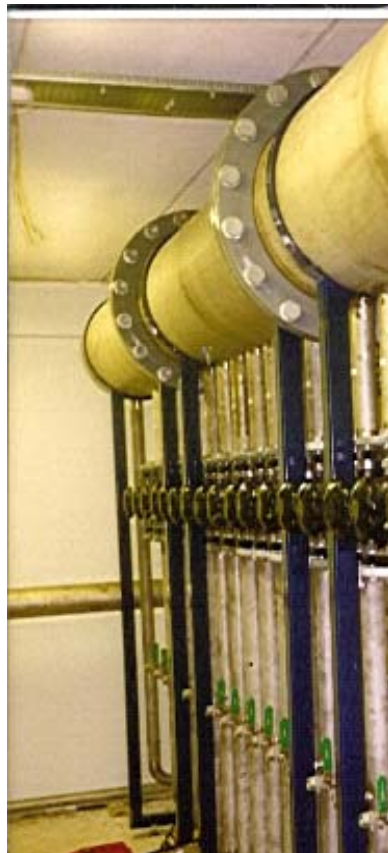
Figure 17. Manifold with diameter 600 mm, gas valves and taps for manual samples. Svartasmoget, Fitjar, Norway
