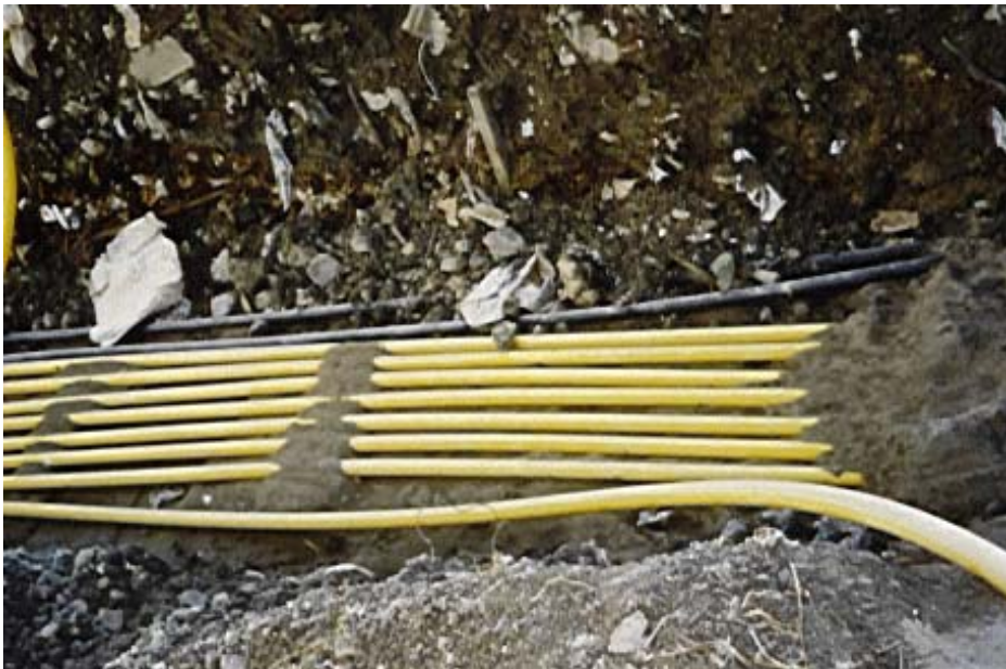
Figure 13. Pipelines (PE63) with underpressure transport LFG from the wells to the collecting station.
