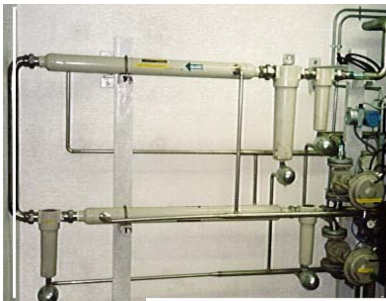
Figure 23. Drying LFG for transportation 40 m below sea level. Seawater is the cooling medium. (Brennevinsmyra, Mandal, Norway)
