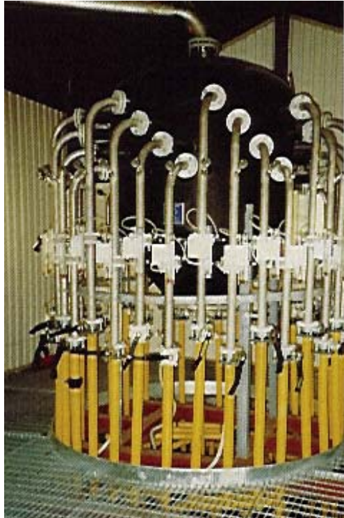
Figure 16. Large volume manifold installed at SVA, Norway
