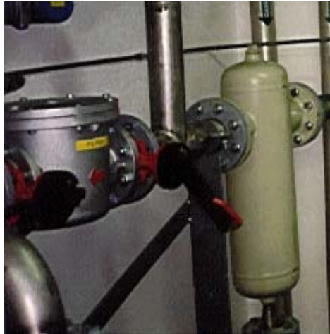
Figure 19. Filter and cyclone to remove excess water and dust/particles (Svatrasmoget, Fitjar, Norway).
