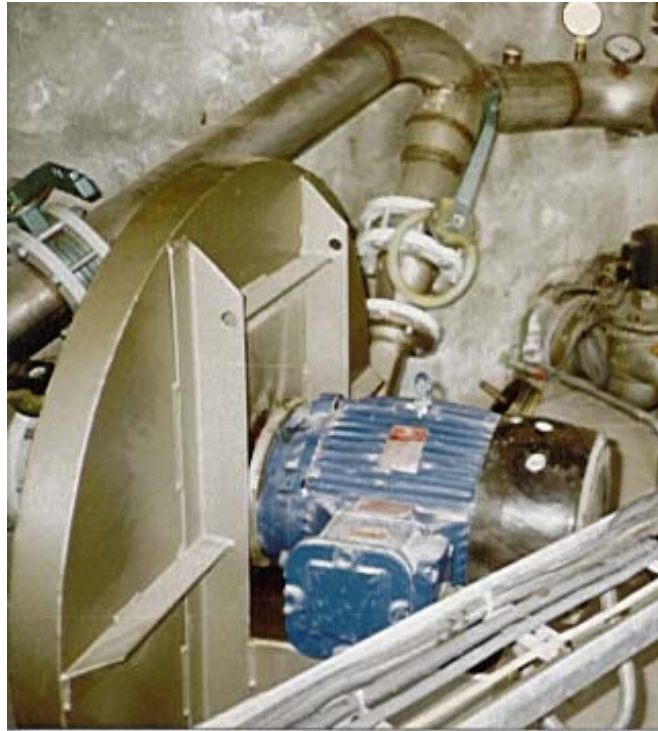
Figure 14. Centrifugal fans were used in early LFG technology (Grinda, Norway).
