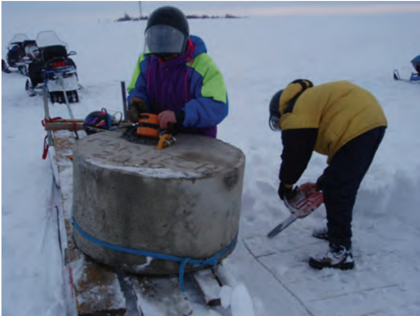
Cutting a hole in the ice to lower the concrete mooring buoy anchor.
